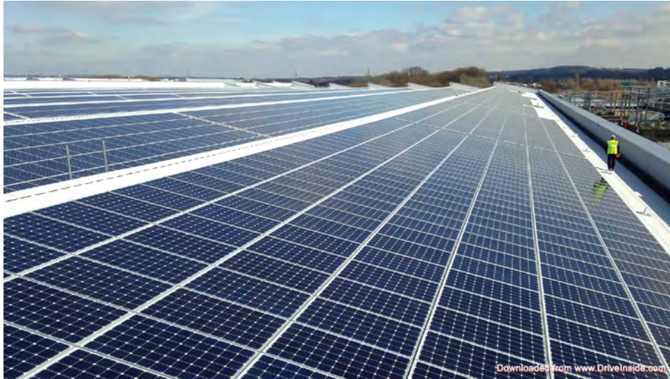
Largest roof top solar array in the world.
